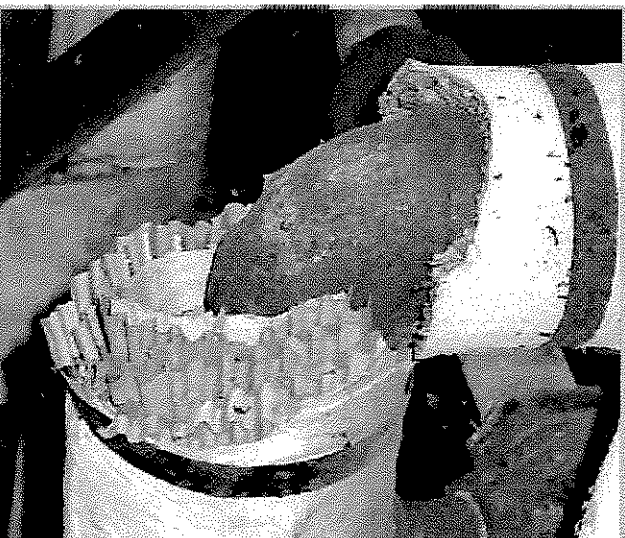
Damaged asbestos pipe insulation.
